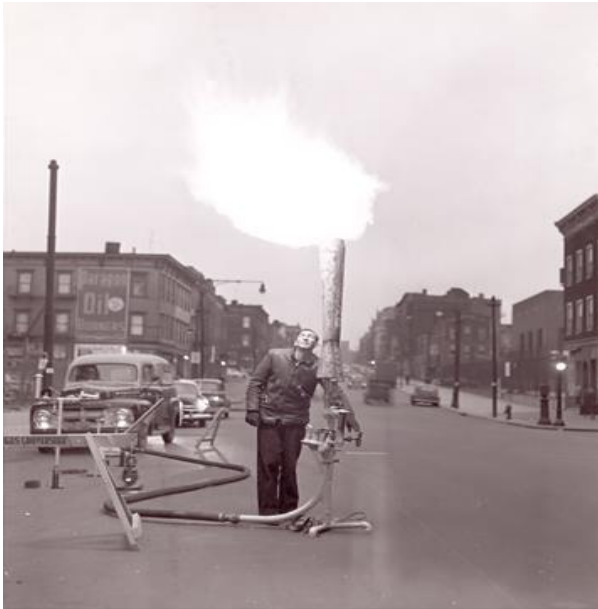
A purge burner igniting manufactured gas being replaced in a main by natural gas during the 'great conversion' in 1952
