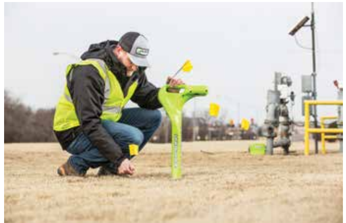
Contractors often use their own personnel to locate and mark buried facilities
