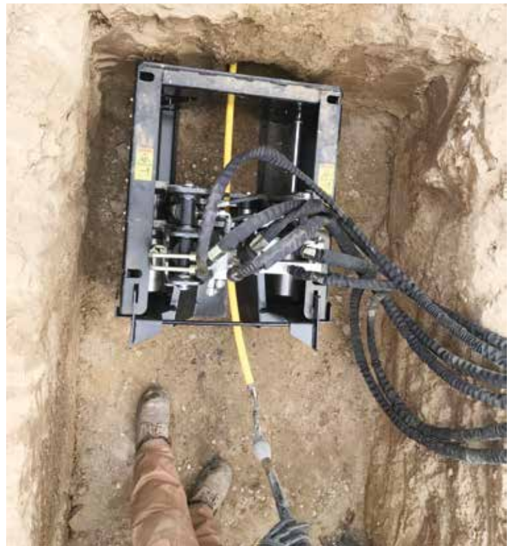
PE product pipe is pulled into place simultaneously as the existing pipe is extracted
