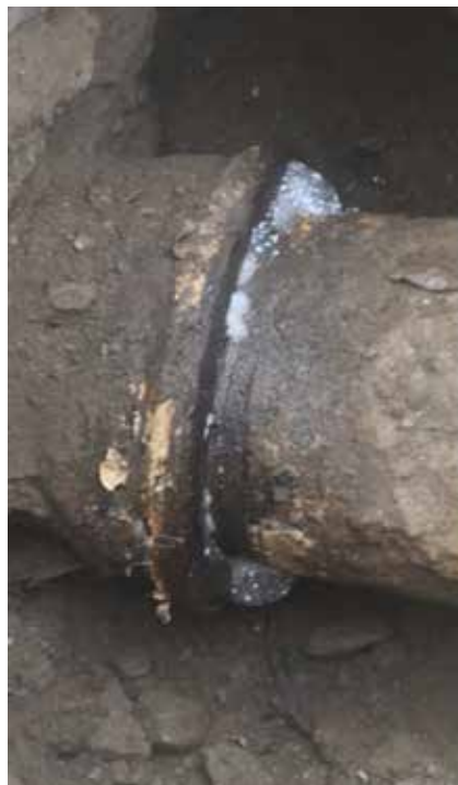
Example of leaking CI joint with leak detection solution applied
