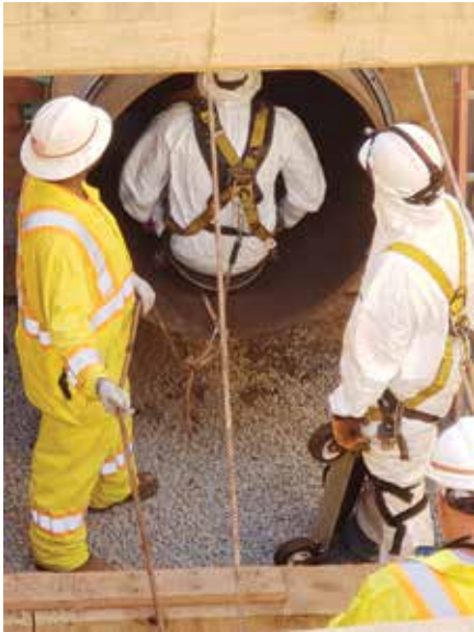
First-ever application of curtain grouting from inside a gas main required man-entry
