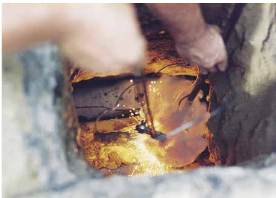
Attaching anode for cathodic protection to steel gas line using cad welding
