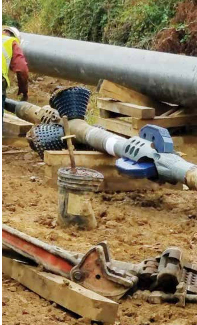
Reducing length of HDD bore path to a minimum can greatly reduce the risk of inadvertent returns
