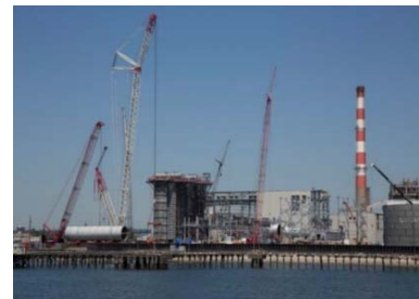
PSEG Power Bridgeport Harbor Station 5 Bridgeport, CT 485 MWs Online June 2019
